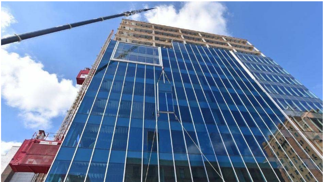
Construction continues on Tower 6 in downtown Allentown on Friday, Sept. 15, 2017. (APRIL GAMIZ / THE MORNING CALL)
